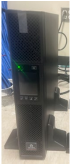
Vertiv GXT5-2000 UPS installed in the 2FL data closet
